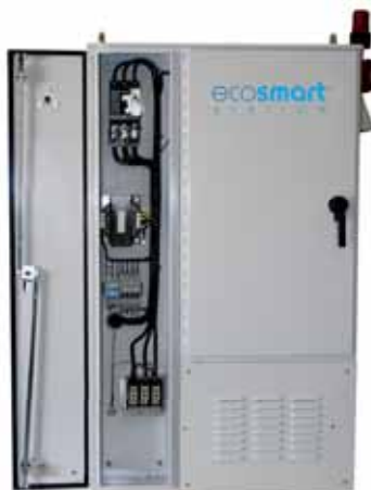
Zone 1: Service Entrance Compartment
