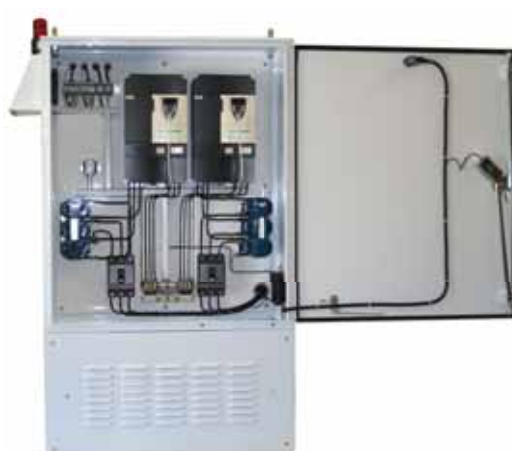
Zone 2: MCC Compartment
