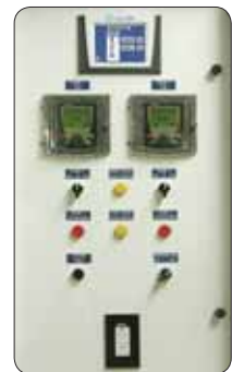
Zone 3: Inner Door of Controls Compartment
